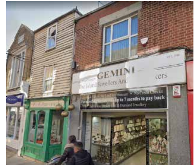
Surviving example of timber framed Weatherboarded upper floor with traditional timber shop front
